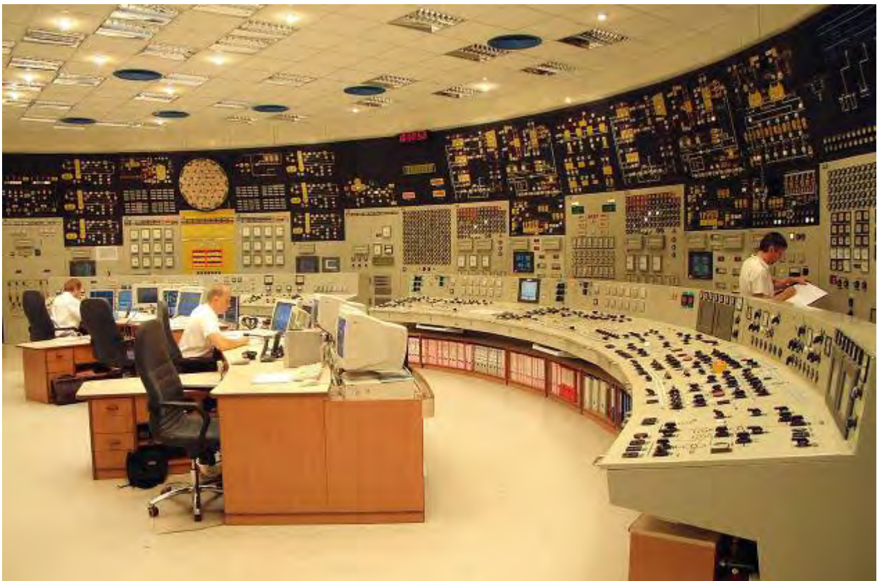
Figure C-12: V1 NPP main control room
