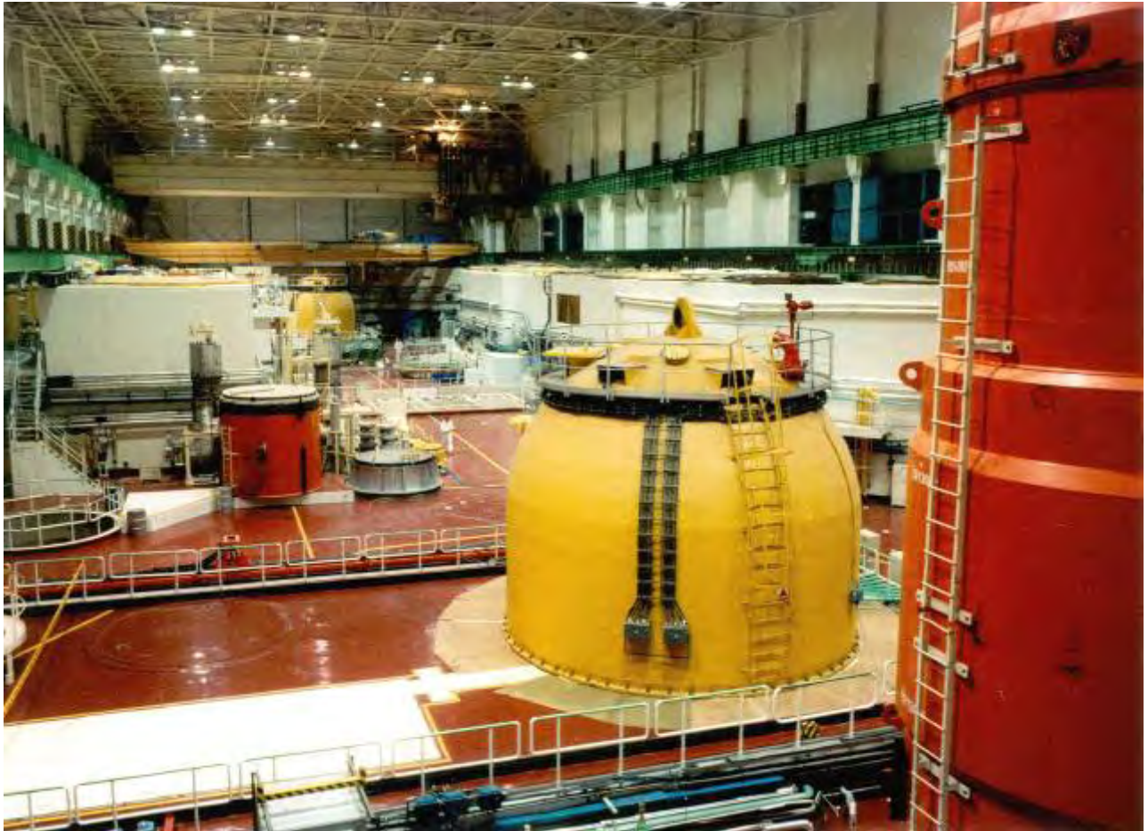
Figure B-1: View of the V1 NPP reactor hall
