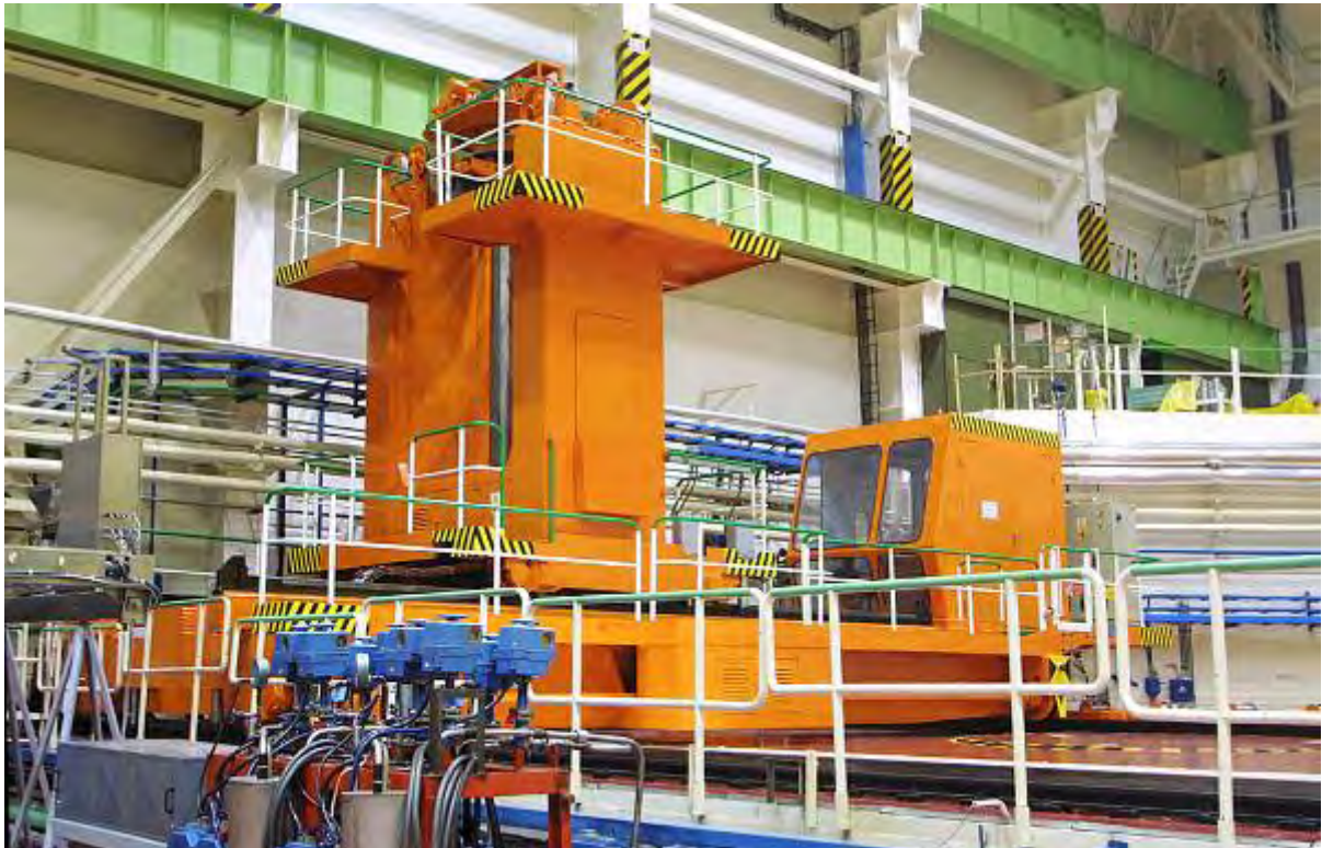
Figure C-11: Fuel reloading machine.
