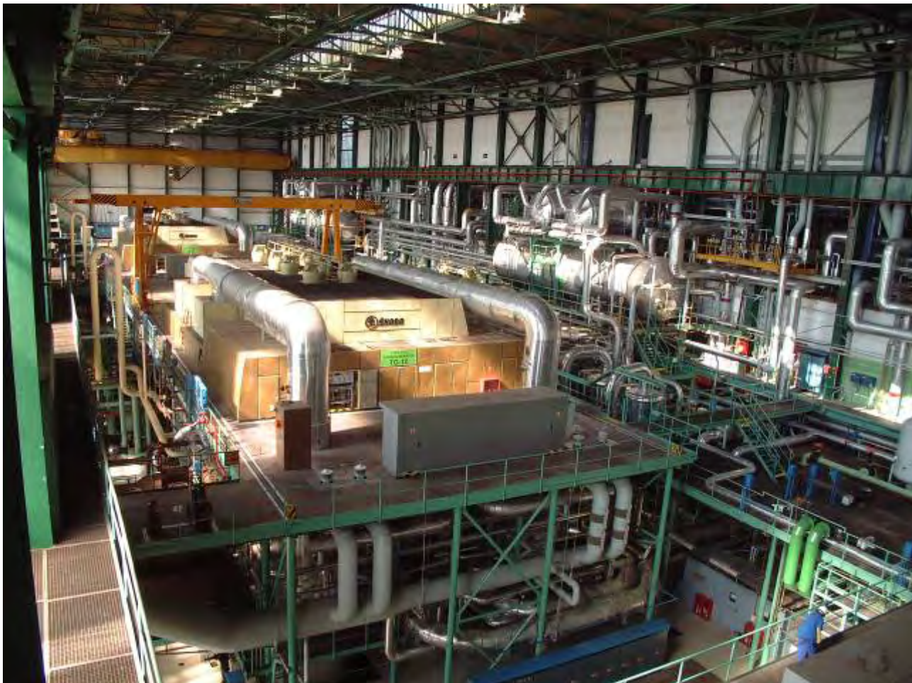
Figure B-2: View of the V1 NPP turbine hall
