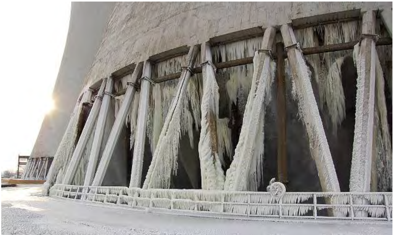
Figure C-10: Cooling tower of the VI NPP during winter time.
